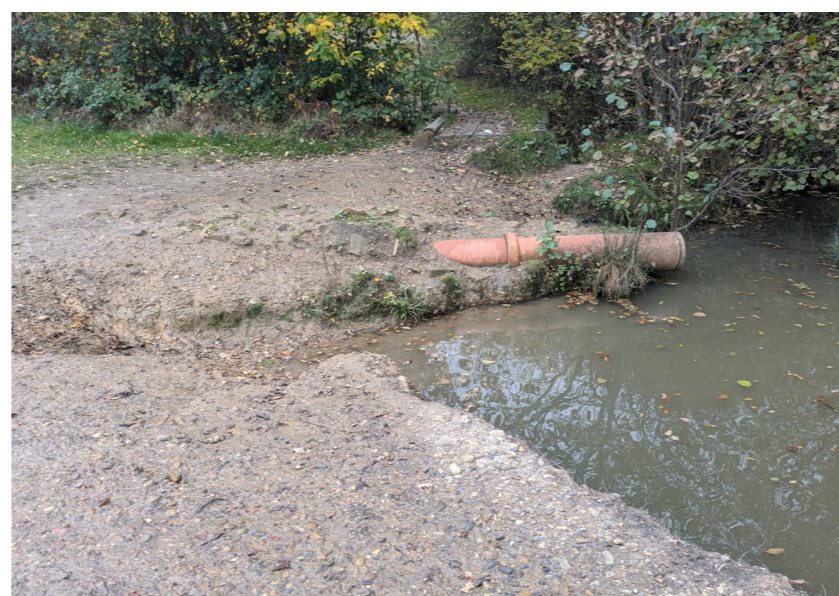
Example of erosion at Trent Park Lake, potential to remove the pipe and create a swale and mini wetland area along with a formalised dog entry area with erosion protection.
